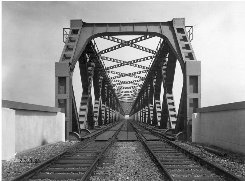
Motif from the RWWA / Railway Bridge Across the Rhine at Wesel (1928) (stock Abt. 130 Gutehoffnungshütte Aktienverein, Oberhausen)
